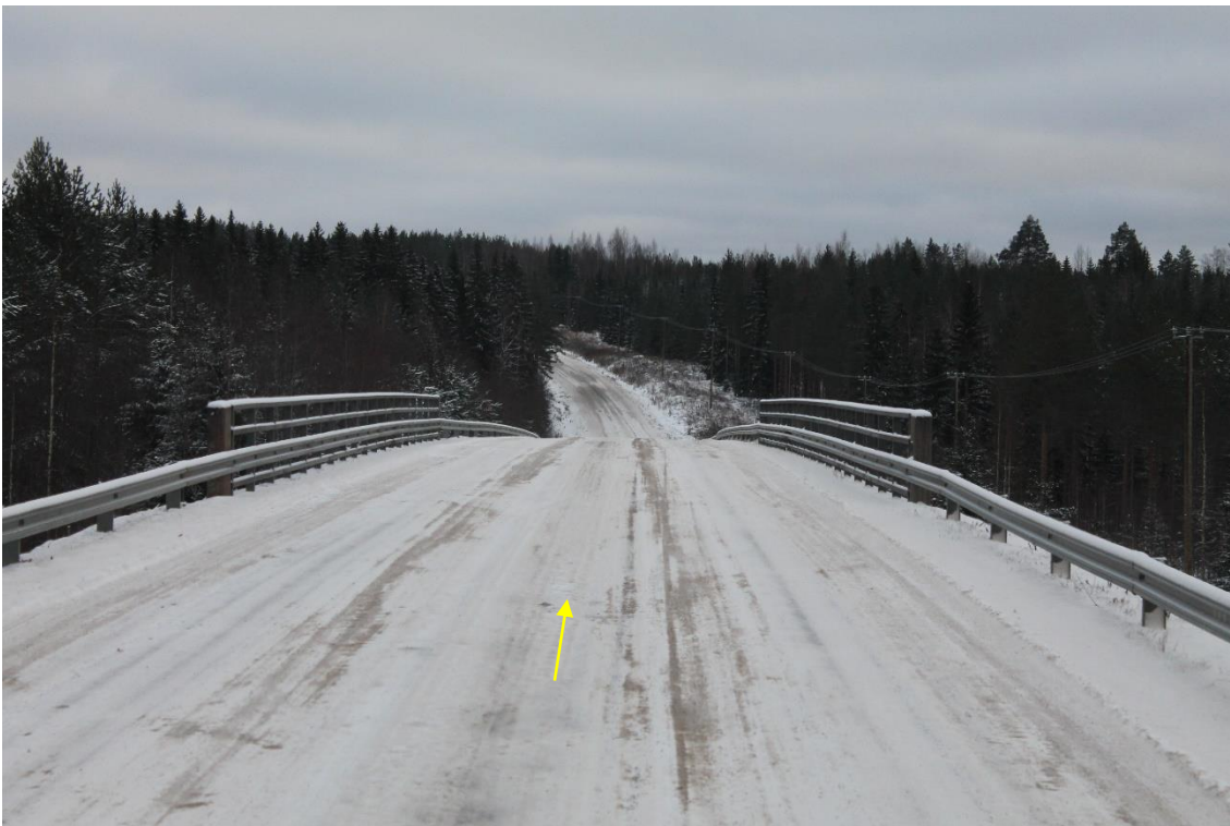
Pos 37/Pic 92. Road 3482. https://maps.app.goo.gl/2tmqXE75pNAjGF9S6 Bridge bearing capacity need to be checked. During the wintertime road need extra maintenance.
