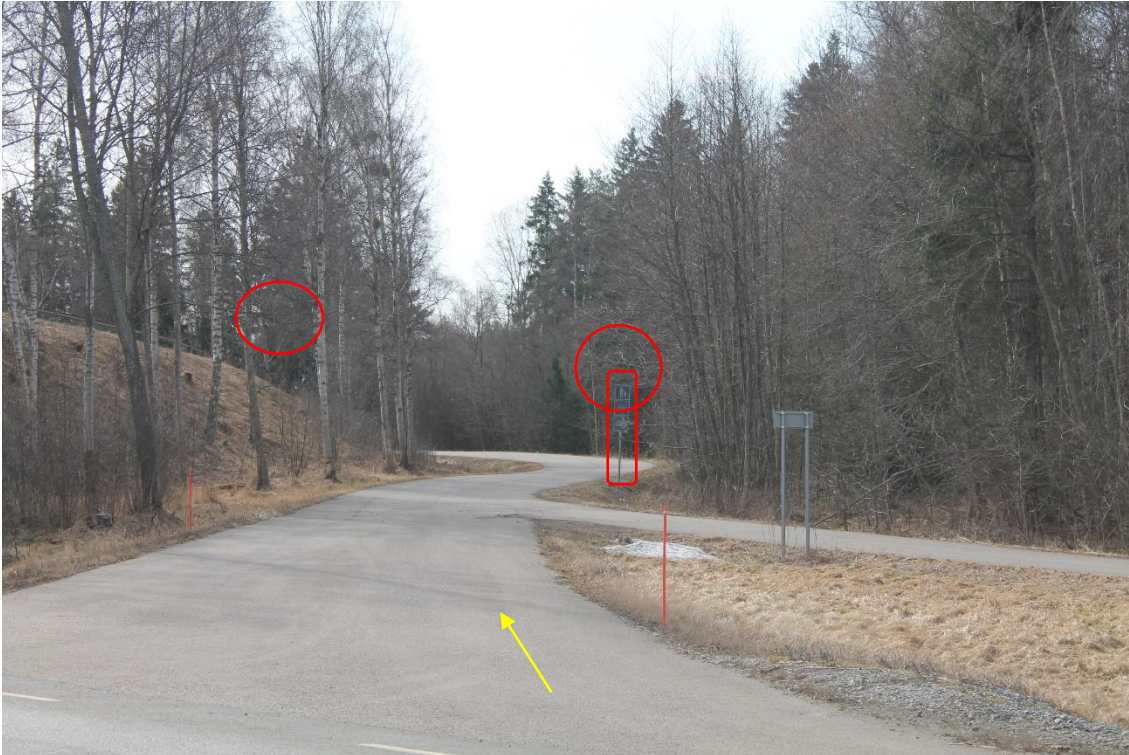
Pos 3/Pic 7. Bridge detour on road 2. Marked sign to be removed. Marked tree branches need to cut.
