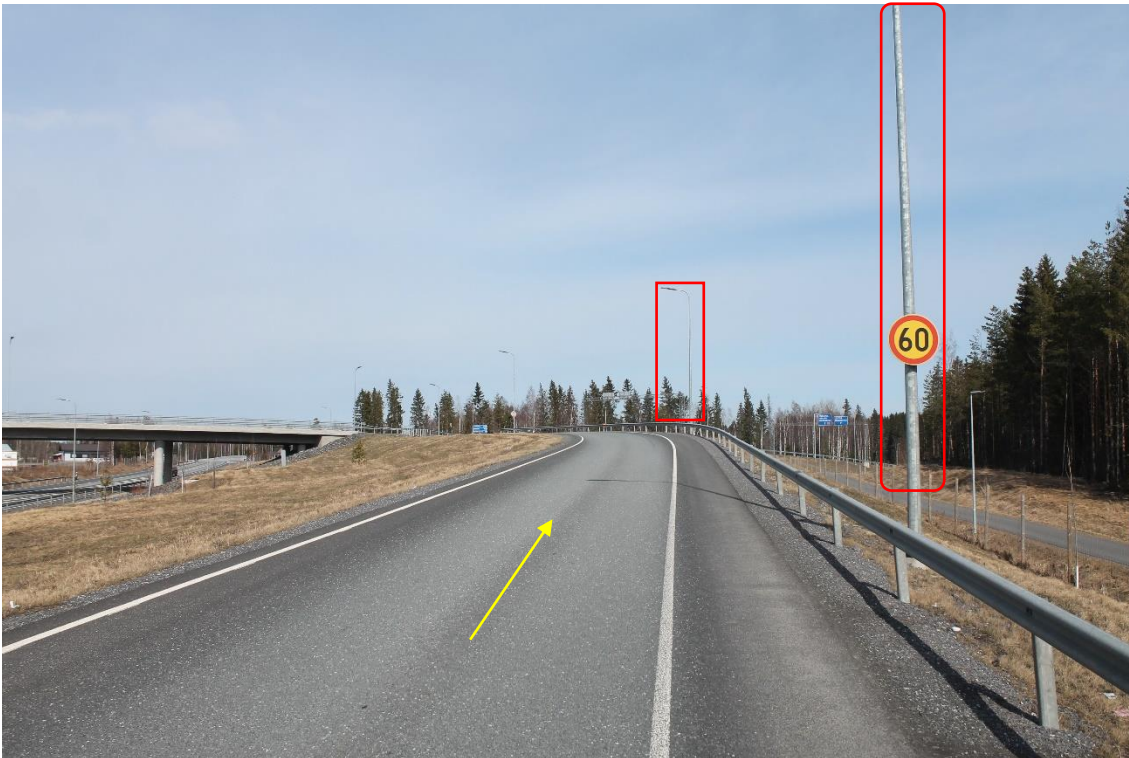
Pos 10/Pic 35. Turning from road 8 toward road 23. Marked lamp posts need to be removed.
