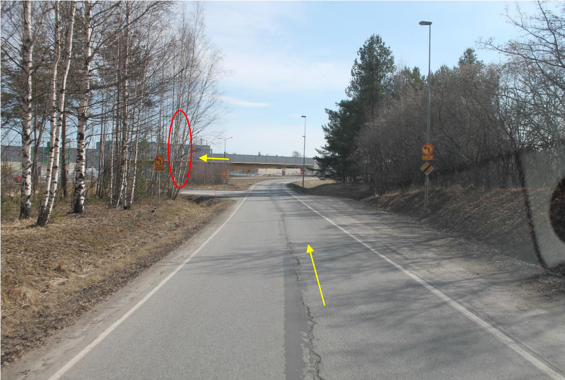
Pos 7/Pic 19. Turning from road 2 toward road 8. Transports need to make u-turn on designed ramp to road 8. Marked trees need to cut. Yellow arrow points driving direction for towers etc.
